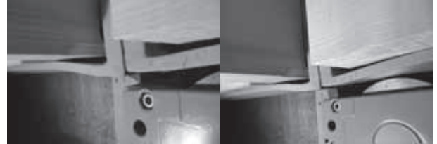
Fig. 7 Example of peripheral beam attachments of rotational platform – view from below, deformation of bottom flanges of peripheral beams
