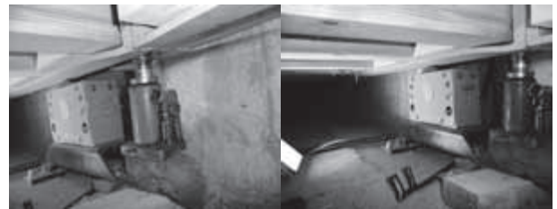
Fig. 8 Deformation of bottom flanges of peripheral beams and modification of peripheral beams connection
